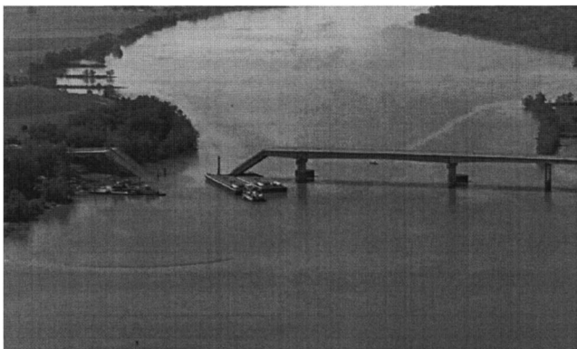
Fig. 2. Overview of damaged I-40 Webbers Falls Bridge
