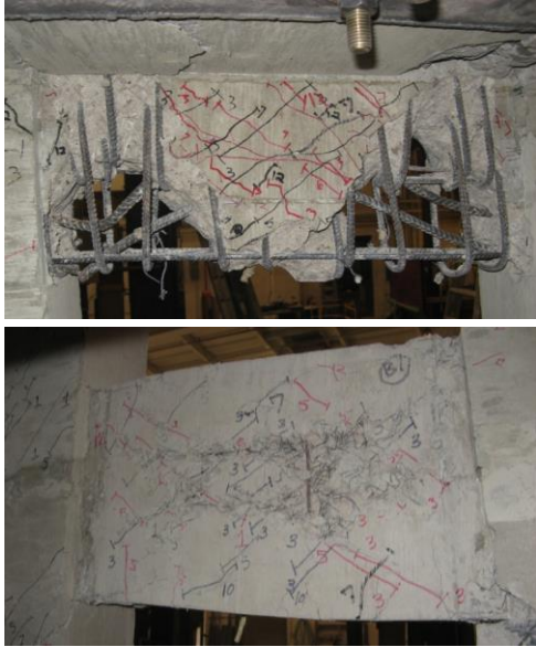
Figure 8. Reinforced concrete (top) and HPFRC (bottom) coupling beams at termination of testing
